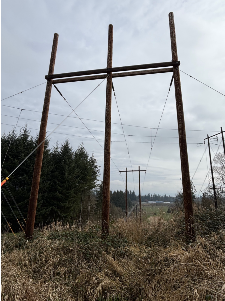
[Current BPA 115kV wooden pole, “H-Frame” transmission towers.]
