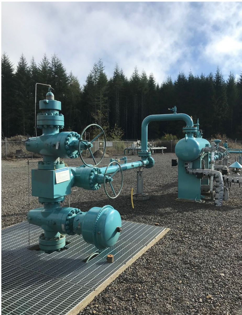
Representative wellhead with moisture and particulates separator in the background
